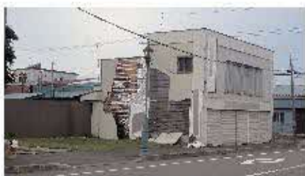
第38図 家屋外壁の崩落(安平町早来). Fig. 38 Collapsed outer wall of a house at Hayakita, Abira Town.
