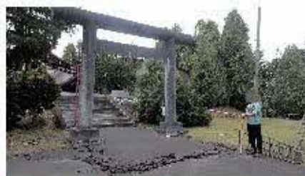
第40図 早来神社における斜面変状(斜面下部)(安平町早来). Fig. 40 Clacks formed at lower side of slope at Hayakita Shrine at Hayakita, Abira Town.
