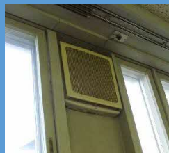
窓設置の換気扇
